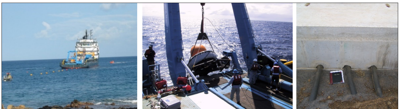
FIGURE 21. HA10 cable landing (left). Node deployment (centre) and detail of cable conduits exiting the onshore splice pit (right).
