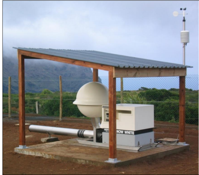
FIGURE 7. A Snow White HVAS situated at RN67.
